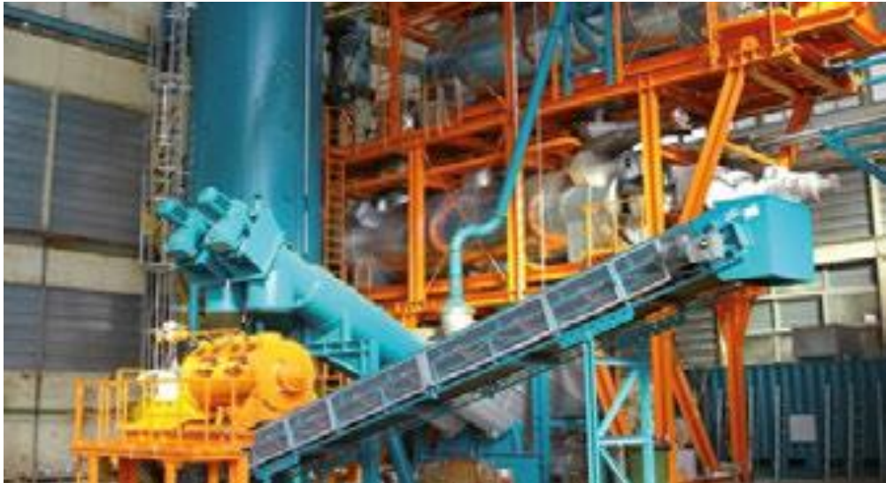
Figure 5 Indirectly heated Vacuum Distillation unit. (Source: econ industries GmbH cited in UNEP/ISWA 2015)
